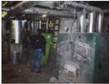
One of original coal boilers
