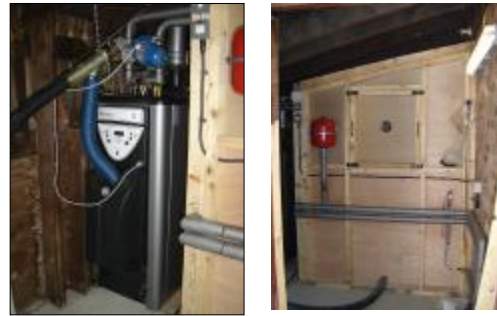
Boiler and fuel store
