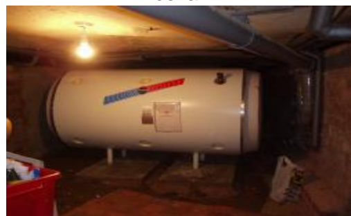
Accumulator Tank in adjacent cellar
