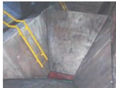
Bunkers modified for wood pellets
