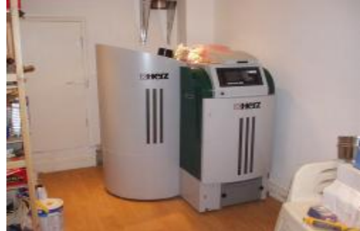
Boiler in utility area.
